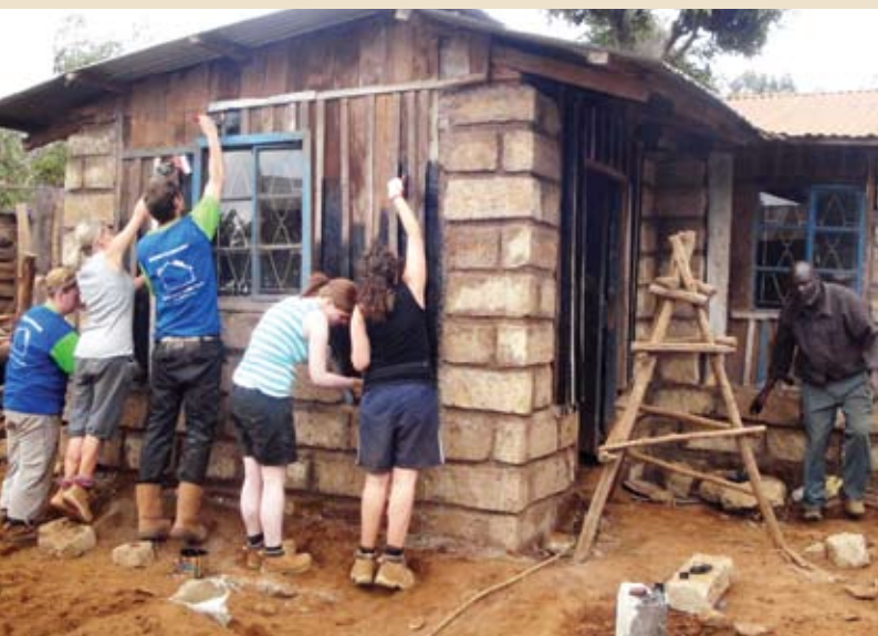
Members of Connie Kwok's team put up a wall for a low income family in Maua.
