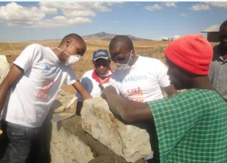
Barclays Bank of Kenya staff put up a wall for a house beneficiary at Maai Mahiu Internally Displaced Housing Project
