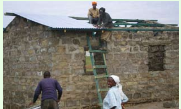
A jovial house beneficiary at HFHK's Internally Displaced Housing Project in Maai Mahiu
