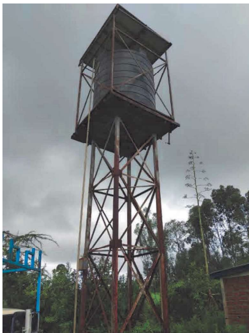
Figure 8: Rusted tank tower
