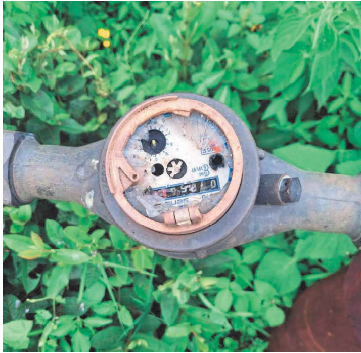
Figure 1: Faulty Borehole Water Meter
